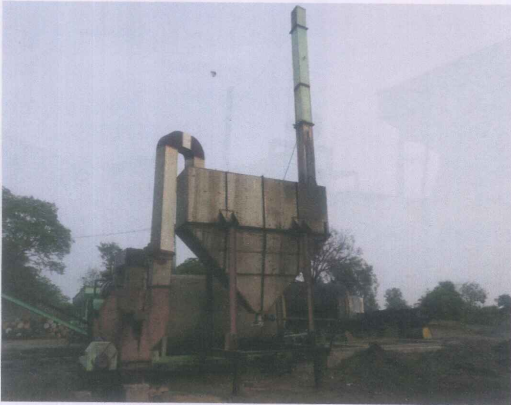
Photographs of M. A. K. Lashmanan Central Hot Mix Plant taken during inspection on 22.8.2022
